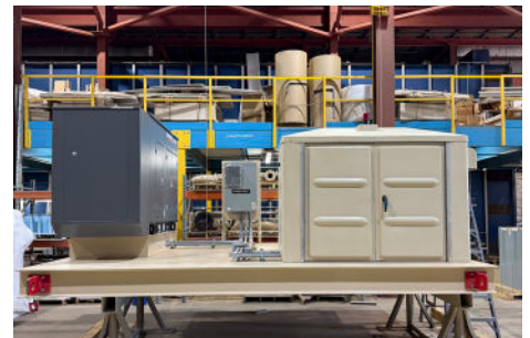
Back-up power generators
