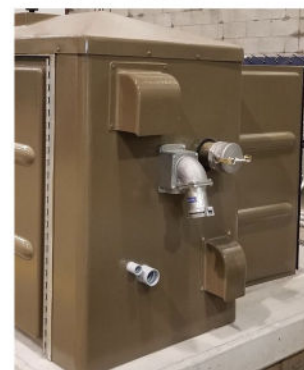
Bypass pump connection & generator receptacle
